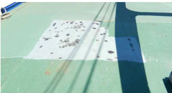
Figure 2 - Example of areas of damage and early progress.
